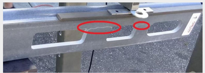
Figure 4.10.4 – Circled break point area image
