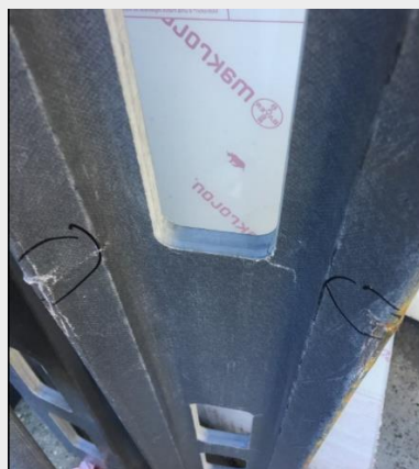
Figure 4.12.4 – Cracks as shown
